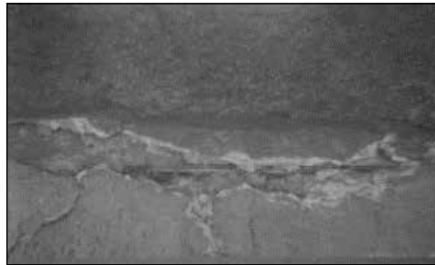
Major Damage to Fire Insulation
